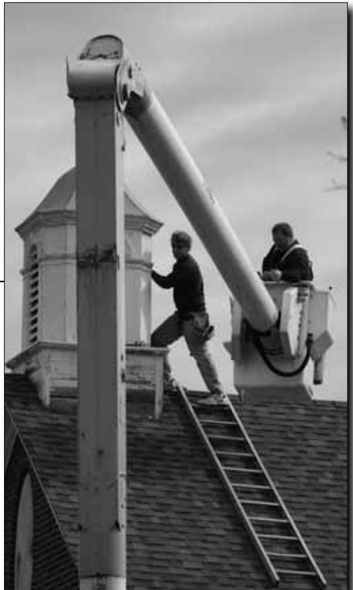
Scooter Tedder and Darin Reid repair the bell tower above the Salisbury Association office.
