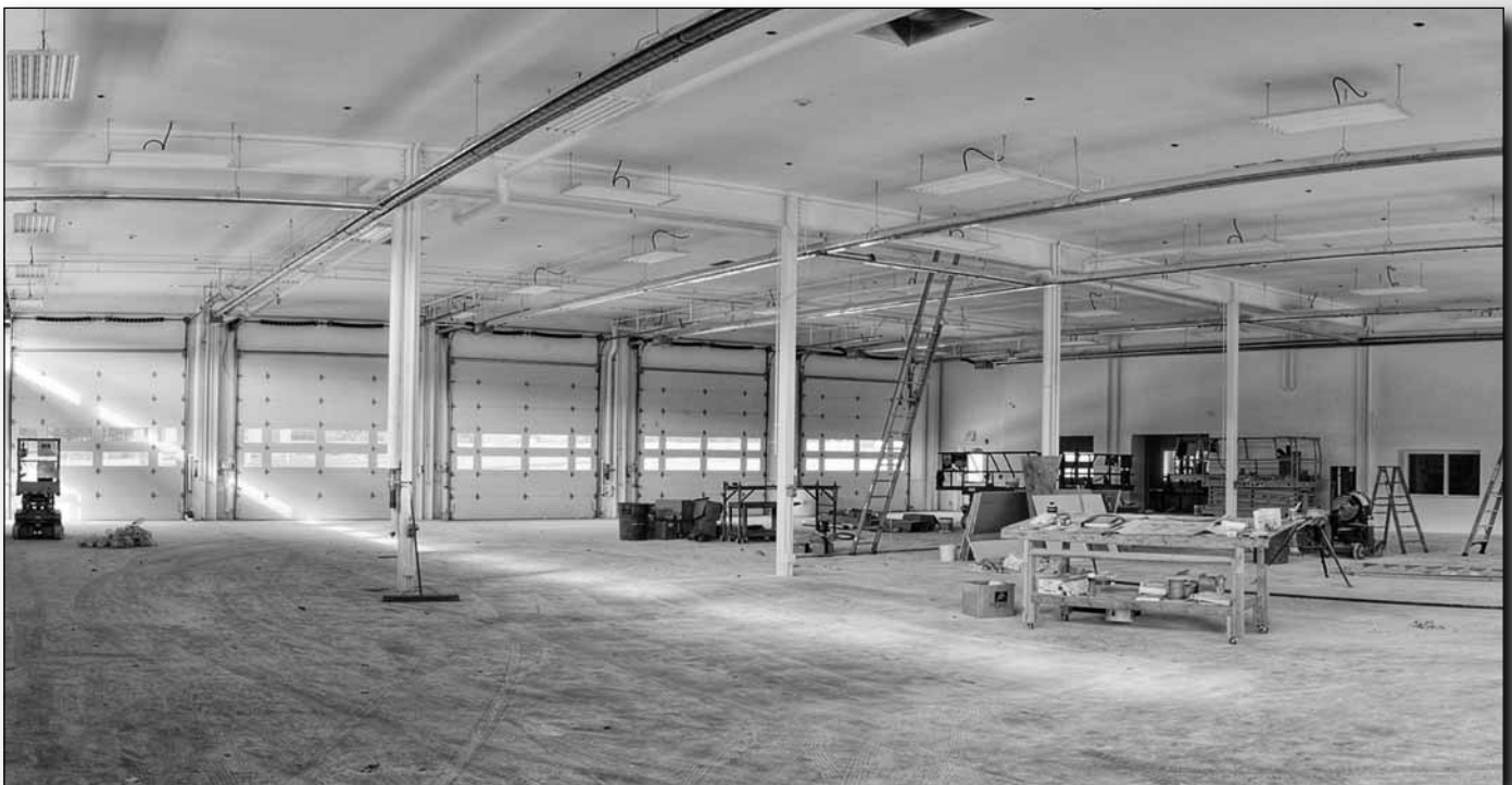
Ready to move in: concrete floors are poured and the fire house is nearly ready for occupation.
