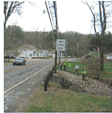
Figure 7. Eroding Roadway at Culvert
