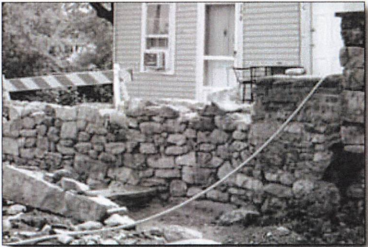
The old stone foundation that was once part of the Holley Block, in Bicentennial Park, was repaired this year.
