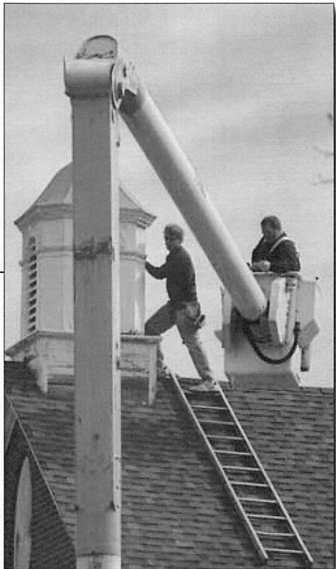
Scooter Tedder and Darin Reid repair the bell tower above the Salisbury Association office.
