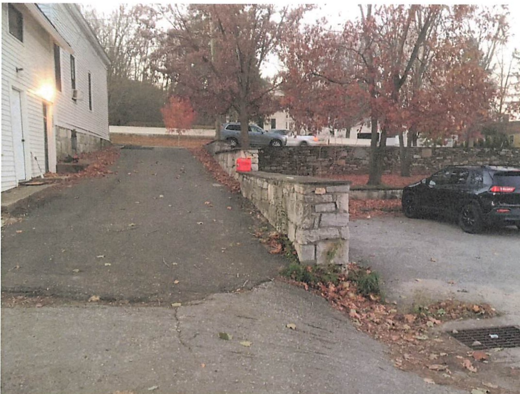
Narrow drive between the commercial building and Holley Block ends in a steep grade and sharp turn
