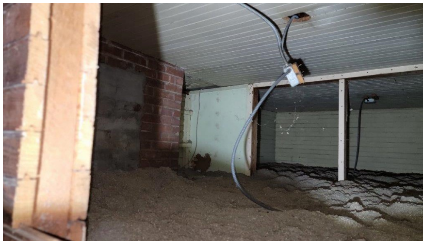
17. Ceiling condition near chimney.
